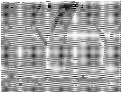
Figure C5: Cracking at base of tread shoulder
